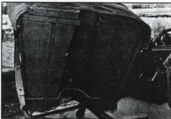
Underside of the body with the new floor and trans tunnel complete.
